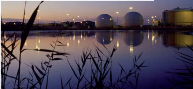
AS AMRA – Jordanie 64.000 m3 de digesteurs
